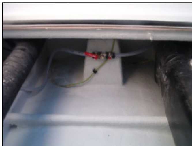
VANNE ALIMENTATION EAU Position of fresh water valve
